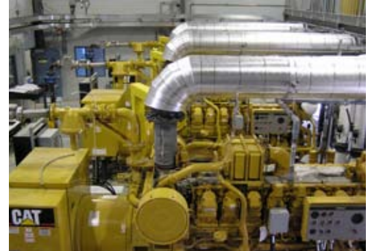
Three Cat® 63516LE gas engines provide enough electricity for about 1,000 customers of Guelph Hydro while reducing pollution emissions from the Eastview Landfill by about 100,000 tons a year.
